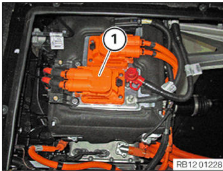
Fig. 324: Identifying High-Voltage Cable Courtesy of BMW OF NORTH AMERICA, INC.
